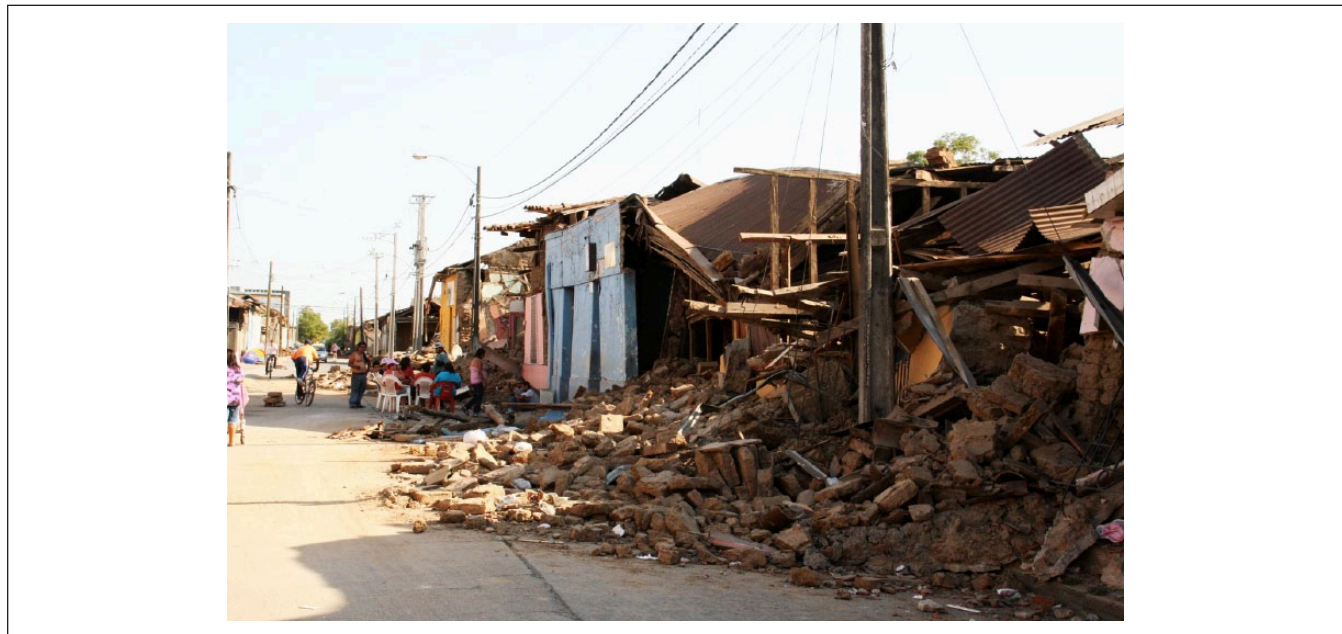
Figure 2. 2010 earthquake damage in Talca. See neighbors living and socializing in the street. Photo: Alexis Martinez.
