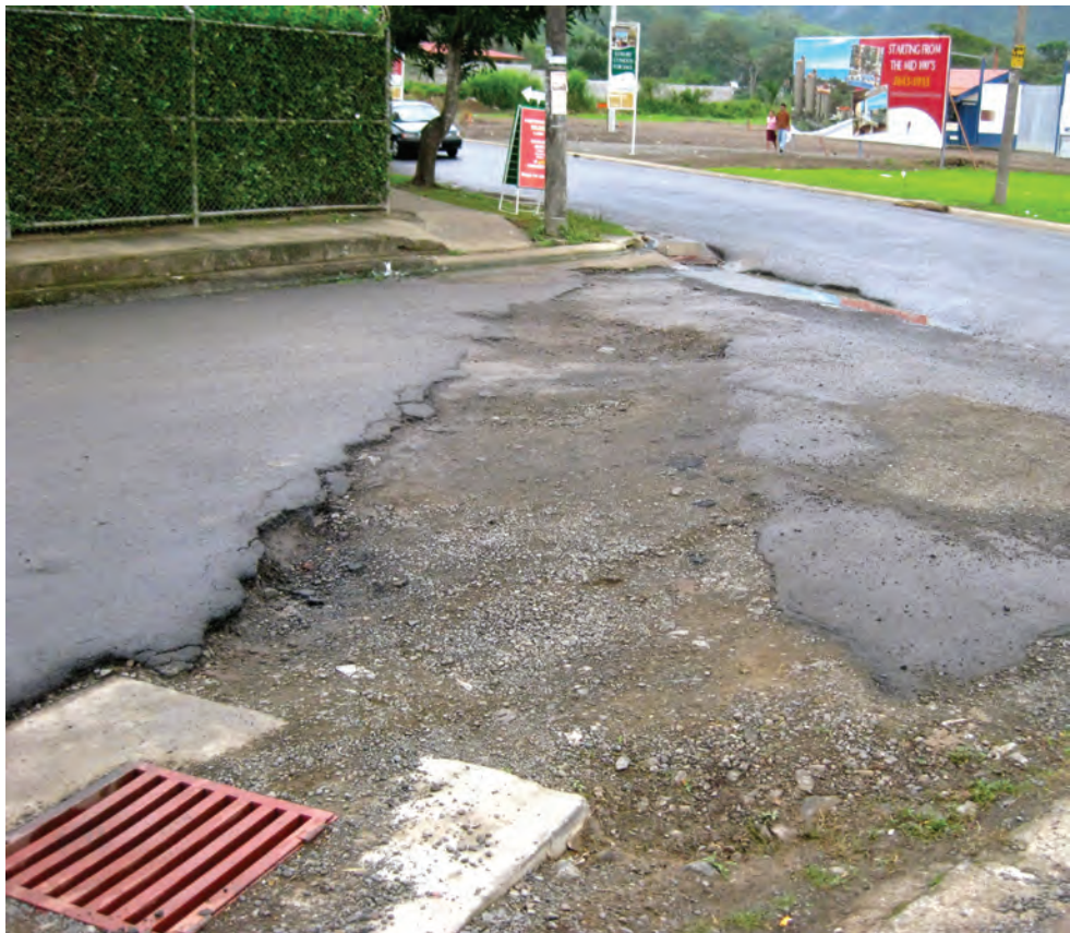
FIGURE 3 Many roads in Jacó are badly maintained or altogether unpaved (photo by Joe Melara, 2010)
